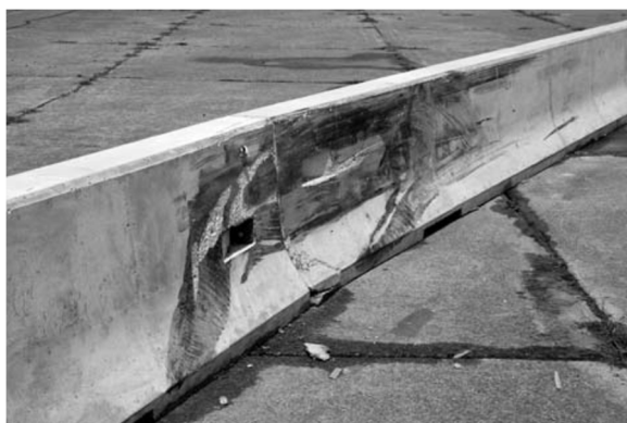
Figure 2.13 Damage to 30-ft long precast barrier with X-Bolt connections ( TTI, 2005 )
