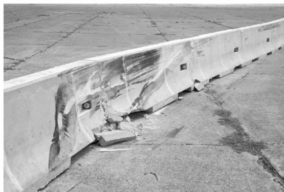
Figure 2.12 Damage to 10-ft long prefabricated barrier with X-Bolt connections ( TTI, 2005 )
