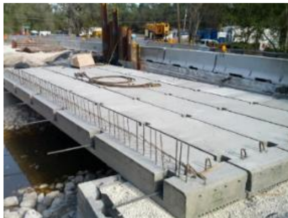
Figure 1.4 Rock Ridge Road bridge with exposed barrier connection reinforcement ( FDOT 2014 Design Training Expo )
