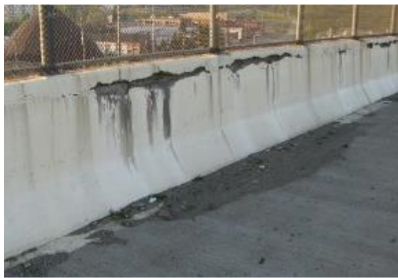
Figure 1.1 Cast-in-place barrier requiring maintenance ( Courtesy of T. Capuano )
