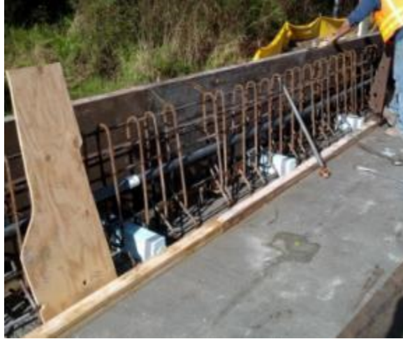
Figure 1.5 Rock Ridge Road barrier after adding additional reinforcing ( FDOT 2014 Design Training Expo )
