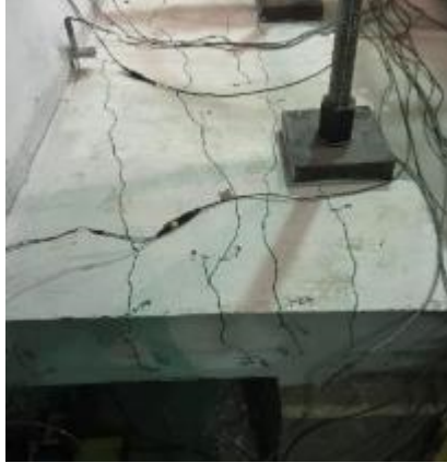
Figure 5.4 Test 1 - Formation of flexural cracks on the deck overhang
